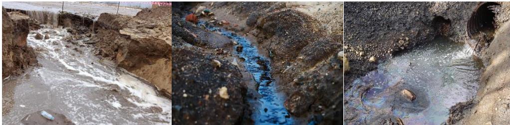
(a) (b) (c) Fig. 2. Impacts on Water Quality (a) Erosion of soil due to disturbed natural slope (b) Leakages of oil and fuel from plant and machinery (c) Waste water accumulating into natural streams
